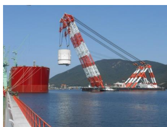
A piece of the 30 storey turret is installed in the substructure lying alongside the quay.
