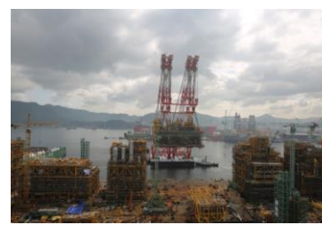
A 4800 tonne gas processing module is lifted from the quay to be carried around and installed on the Prelude facility.
